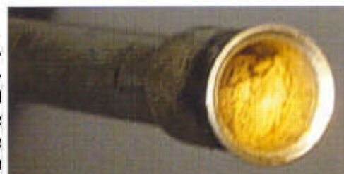
End view of an evaporator neck shows why there was no cooling. The evaporator is plugged with hardened sealer.
